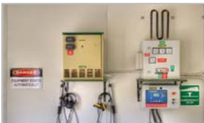
IMG10: Constant volt charger (left) and turbine controller (right)
