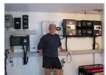
IMG5: THE ELECTRICAL CONTROL ROOM
